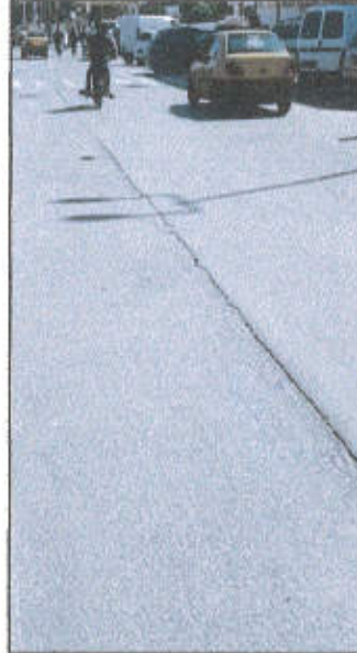
Fissure de joint
